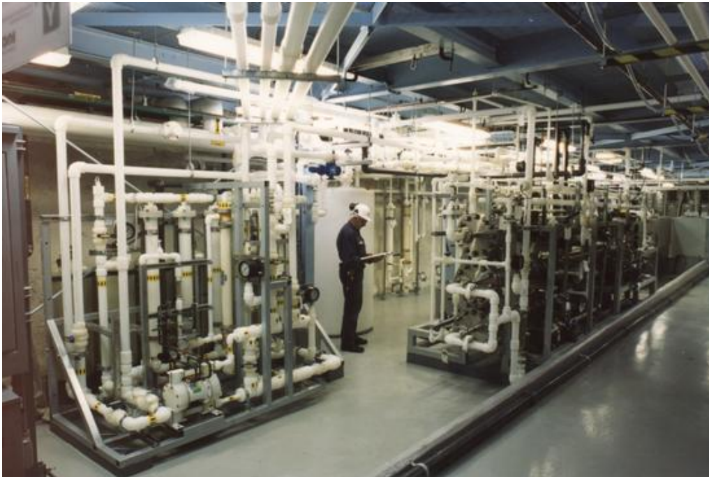
Figure 5.2: Part of the SNO water systems. The feed/bleed tank can be seen (centre) and some of the recirculation pipes.
